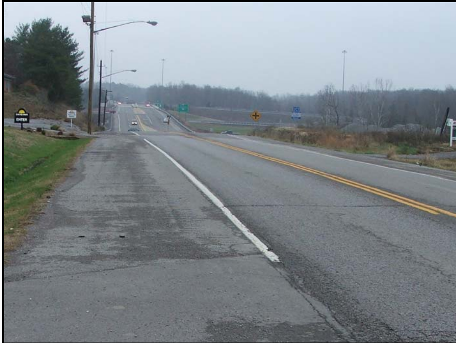
Approaching parkway from north near transition from 2-lane to 4-lane section at Location 2-A
